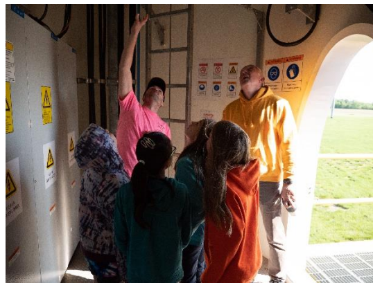
The inside of the turbine is always the most interesting part!
