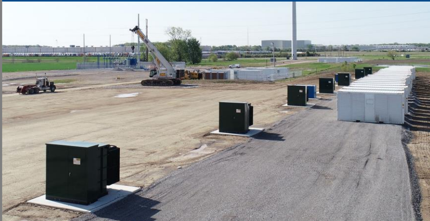
One Power Megawatt Hub site - Findlay, OH
