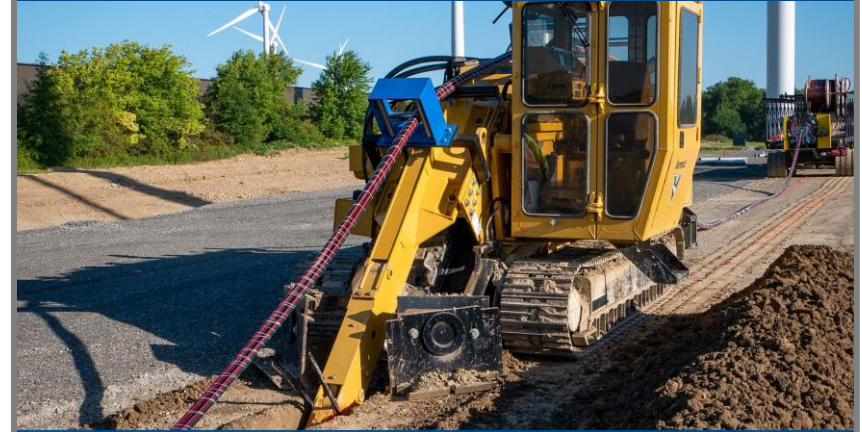
One Power ManagedHV installation - Findlay, OH
