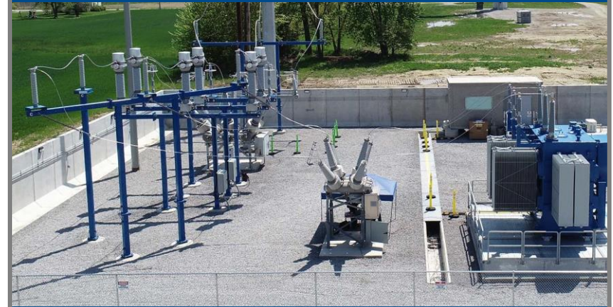
One Power digital substation - Findlay, OH
