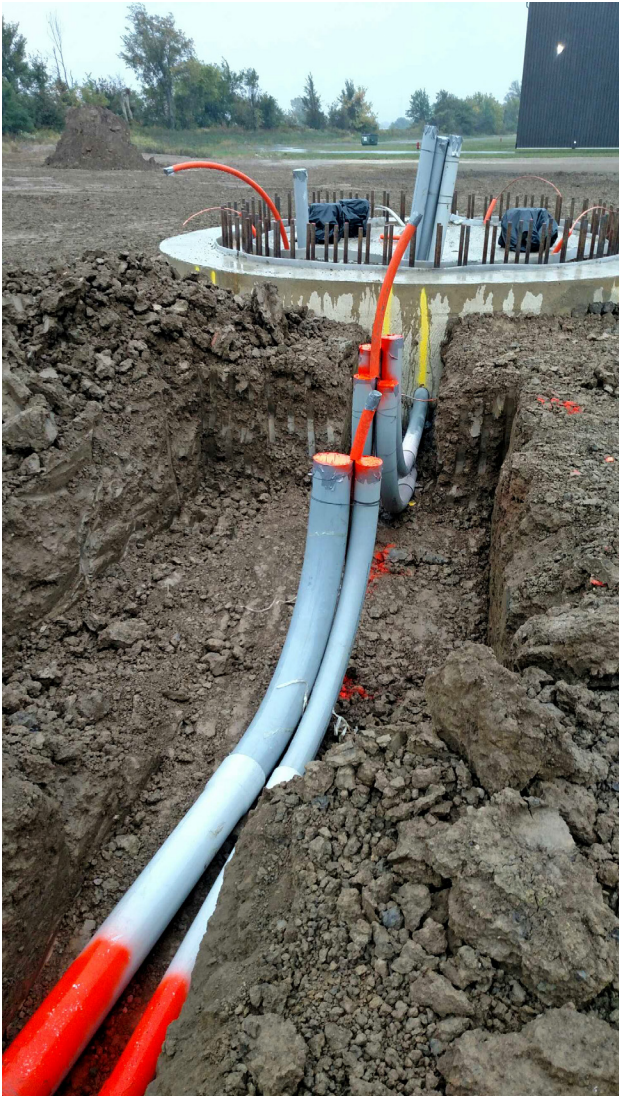
A trench is excavated below the turbine foundation for the low voltage conduit. Electrical conduits are installed in the trench and backfilled.
