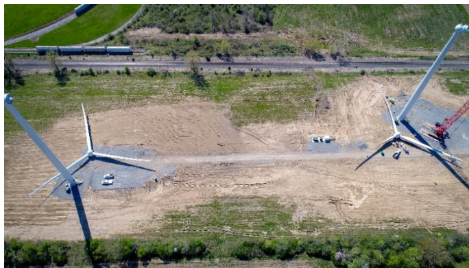
A drone shot of two constructed rotors before they are brought up to the top of the tower.
