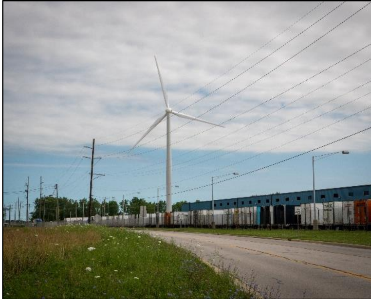
A 1.5 MW wind turbine.
